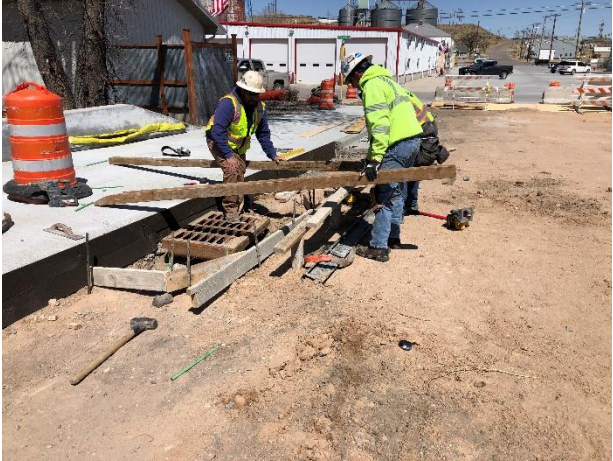
Rough setting of new inlet grate on west side of new concrete box @ Republican River
