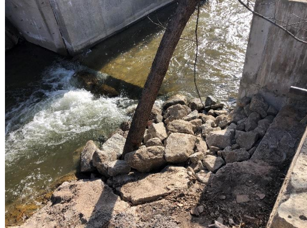
Installation and placement of additional RIP-RAP at downstream outfall of Republican River
